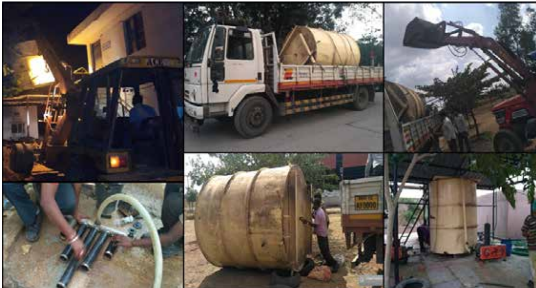
Improved Sequential Batch Reactor (SBR) for wastewater treatment
