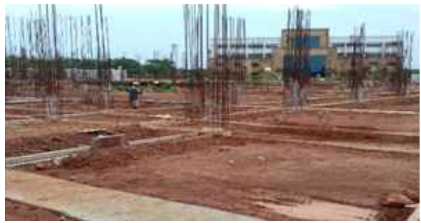
SEOCS: PCC for plinth beam base work and earth filling are in progress.
