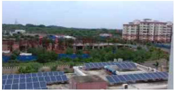
Type-B3 & B4 Quarters: Ground floor slab completed in B4 and B3 column work is in progress.
