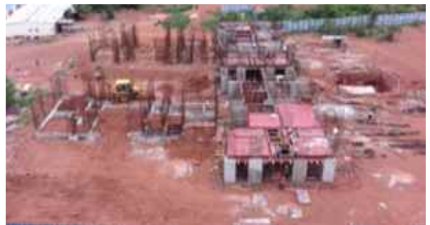
D Type Quarters: Front side roof slab shuttering work is in progress.
