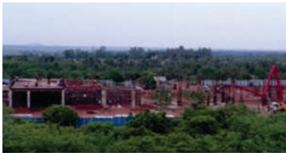
Central Workshop: Roof slab shuttering and column casting work is in progress.
