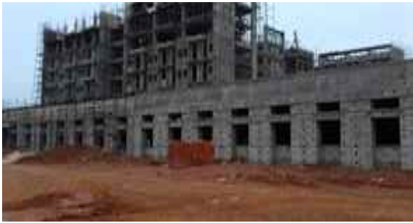
Boys' Hostel-2: A wing 7th floor column work is in progress and roof beam shuttering work is in progress. Block work 2nd floor is in progress.
