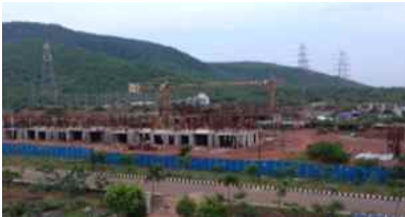
Type-B1 & B2 Quarters: Ground floor slab completed. Column work is in progress in first floor.
