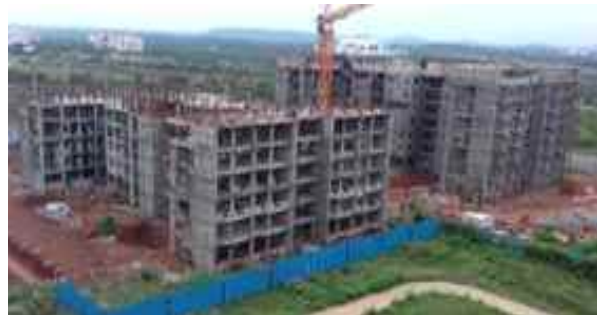
Girls' Hostel- 2: B wing back side 6th floor slab completed& Front side column work in 6th floor slab is in progress.
