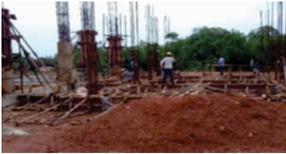
HSSM : Plinth beam work and column above plinth beam work is in progress.
