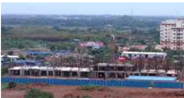
Type- A1 & A2 Quarters: Front side ground floor slab completed. Column work is in progress.
