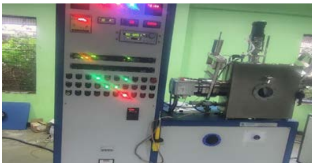
Newly installed Electron beam evaporation system in Microelectronics Lab
