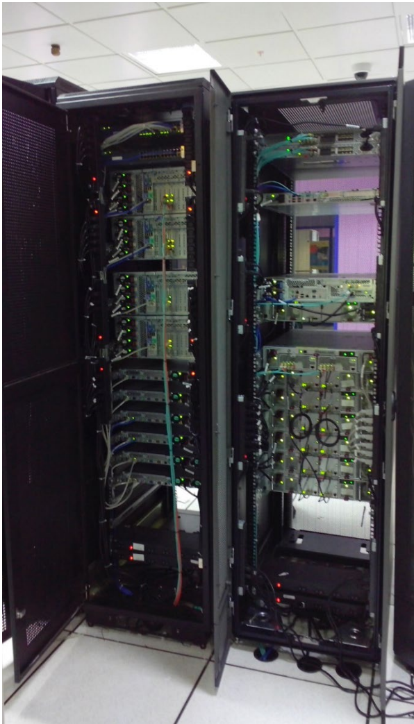
Exchange server: Front view
