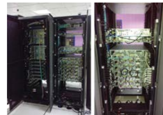
Exchange server: Front view / Exchange server: Rear view
