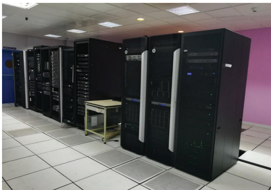
E-Services server area in the data centre
