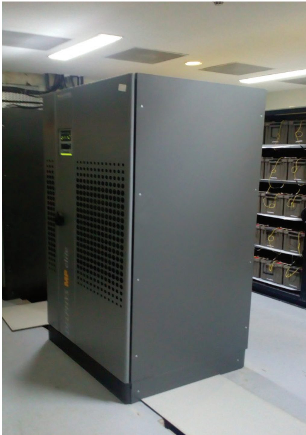
Newly installed 200 kVA UPS
