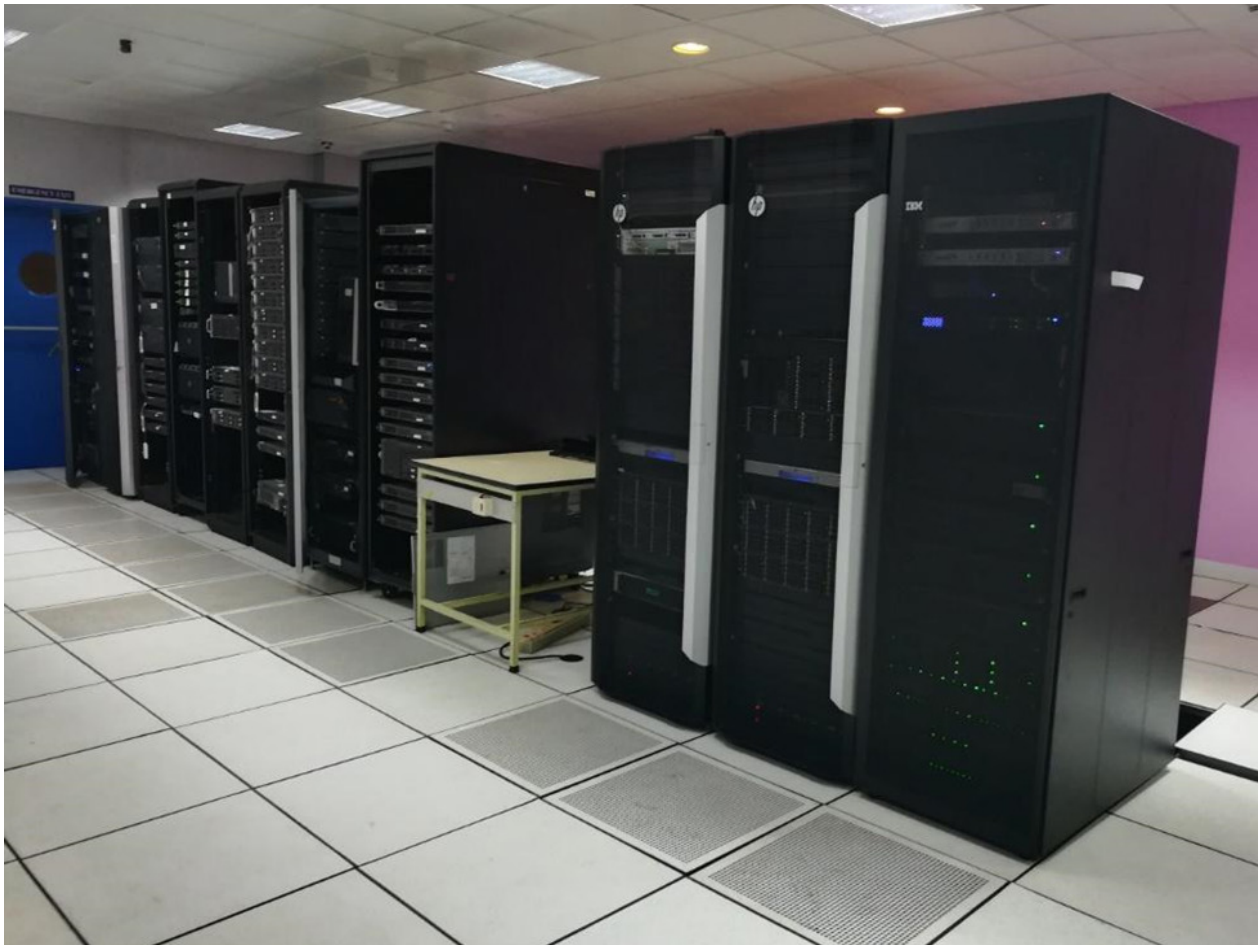
E-Services Server Area in Data Center
