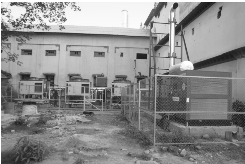
Photograph 8: Side view of newly constructed Supercomputer sub-station
