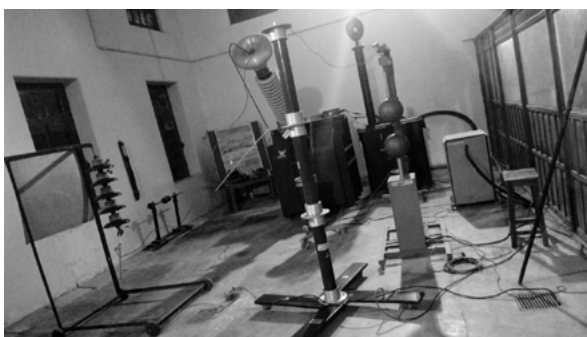
High Voltage Lab
