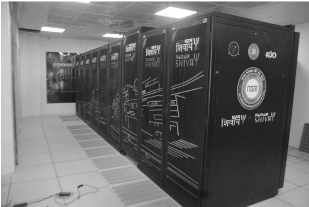
Photograph 9: Establishment of Supercomputer “Param Shivay” (inside Supercomputing building)
