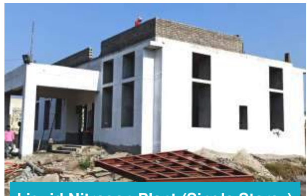
Liquid Nitrogen Plant (Single Storey)
